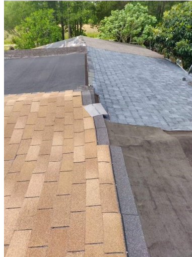
Patchwork roof before (Above)
